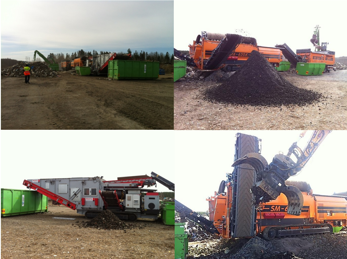
Figure 4. Initial piles with mixed waste and individual piles of the mechanic separation. Image to the right shows the magnetic separation of small pieces of metals from soil fraction.
