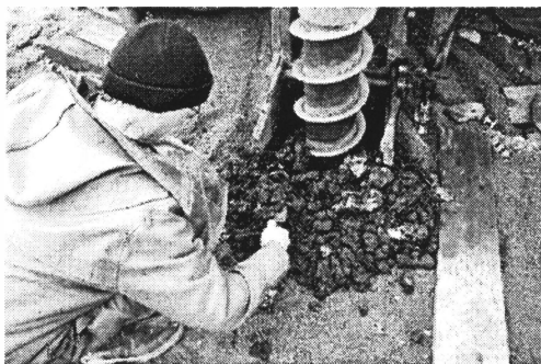
Picture 1: A drilling machine takes up old waste materials from different depth levels (the picture is from the Högbytorp landfill, Stockholm, Sweden).
